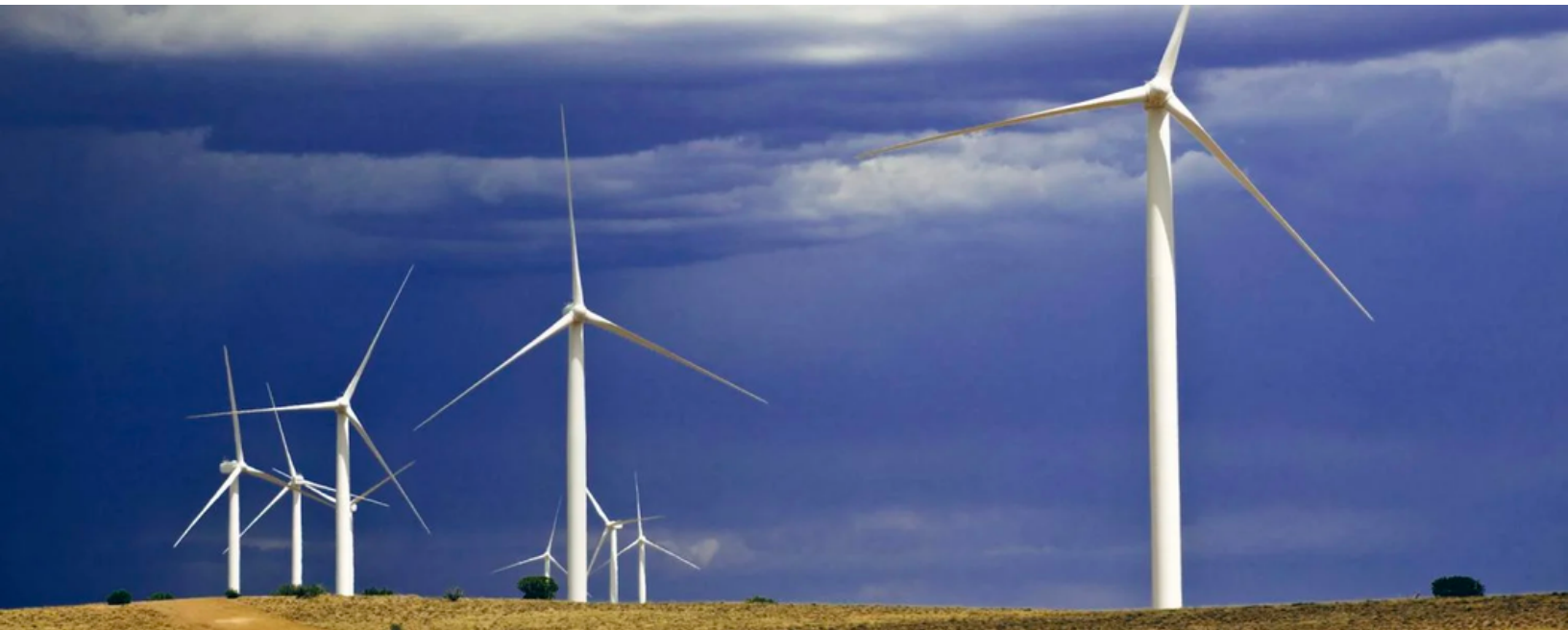
Boulder, Colorado wind farm
